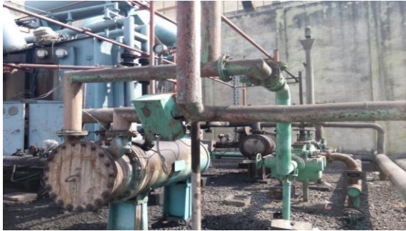
Transformation GRT cooler CSTPS Chandrapur
