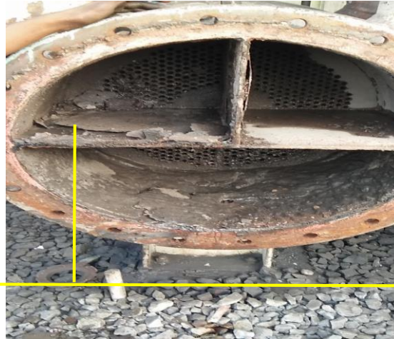
Scales inside the GRT Cooler (heat exchanger) before treatment
