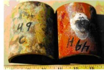
Tube showing localized bulging at hot side (right)
